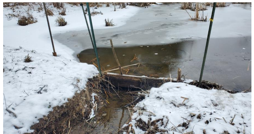
Figure 7. Spillway/stop logs installed at the south end of the impoundment by the landowner to help maintain water levels below the elevation of Lyman Road to prevent overtopping. February, 2023.
