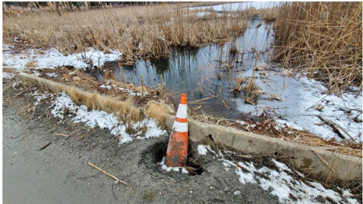
Figure 5. Looking downstream toward the impoundment at Lyman Road, February 22, 2023. Note the sinkhole at the existing road-stream crossing.
