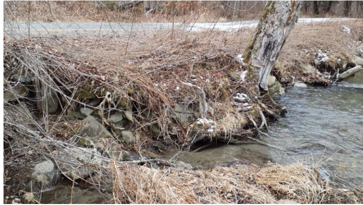
Figure 13. View of the intact impoundment with approximately four feet of freeboard between the impoundment and roadway. February 2023.
