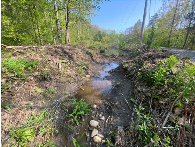
Figure 10. View of the overflow/diversion channel that has been dug to direct water from the impoundment south along E. River Road to an existing stream. May, 2023.
