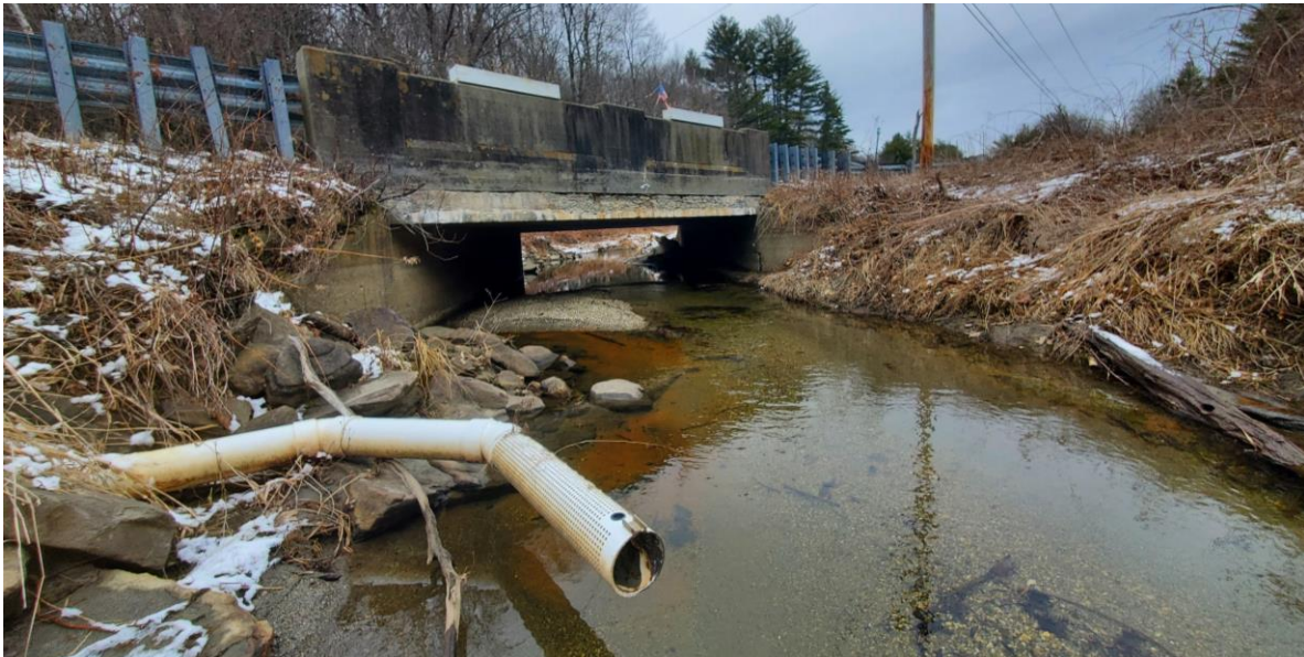
Figure 18. The exposed dry hydrant at the crossing of Skyline Trail and Roaring Brook no longer offers fire protection as it does not reach the water. February 2023.
